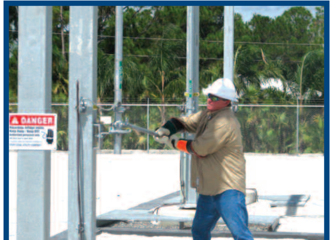
John Dean, Northern District Line Superintendent, closes the load side disconnect switch
